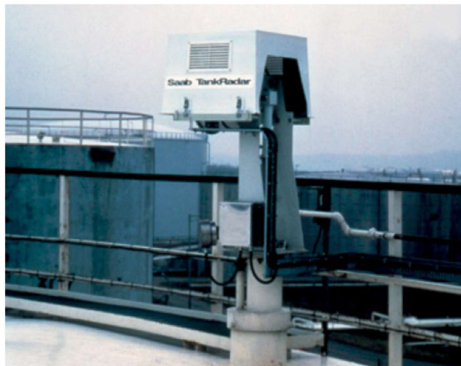
Figure 11: First high precision radar gauge installed in 1985 on a refinery tank
