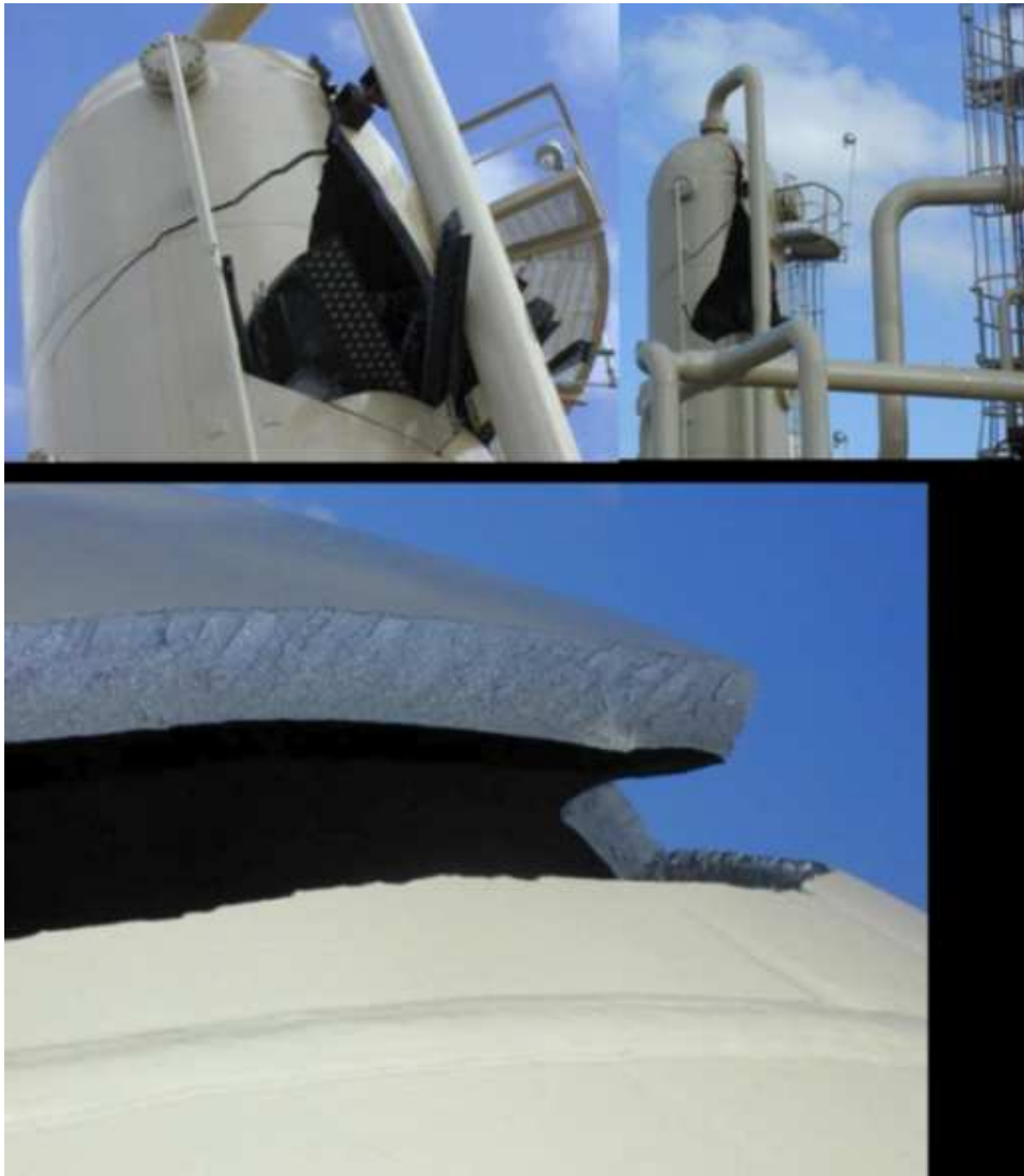
Figure 2. An example of fracturing in a vessel made from the SA-212B Firebox steel.
